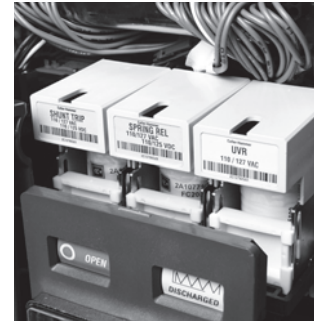
Shunt Trip, Spring Release and Undervoltage Release Device Installed on Accessory Deck
